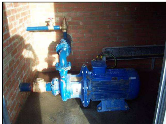
Fig 30. Lowara High Pressure water pump with 55kW Motor and Pressure Relief Valve
